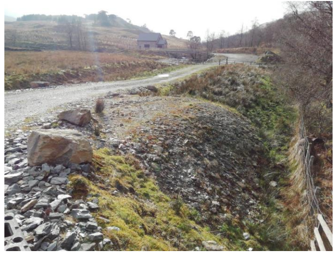
Figure 18. Upper Falloch: facing southwest, shows sparsely revegetating. In the middle distance, water pooling is evident, resulting in gravel bleeding into the far verge due to runoff; viewpoint 6
