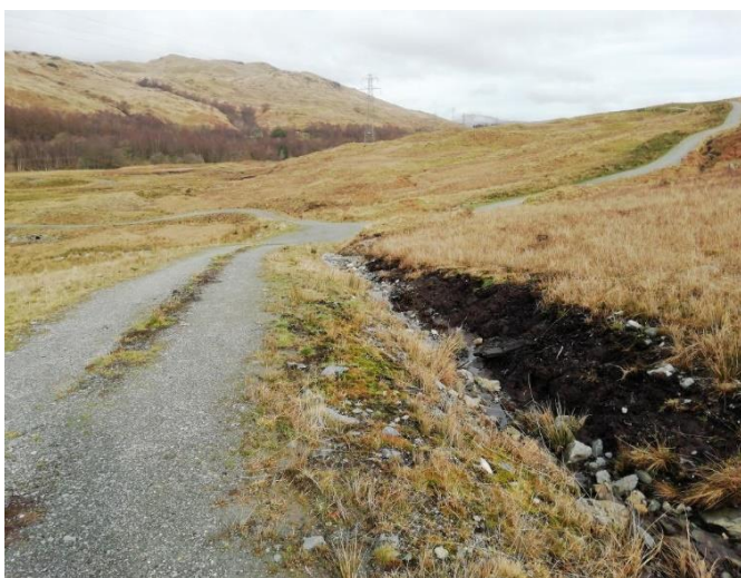
Figure 10. Derrydarroch: exposed soil on intake 4's track. Facing northwest towards existing tracks with the track for intake 2 visible in the distance; viewpoint 4
